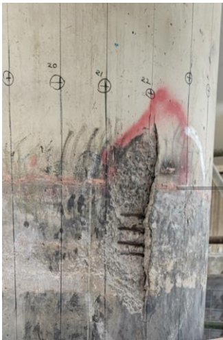
Photo of Column 5 with spalled concrete
