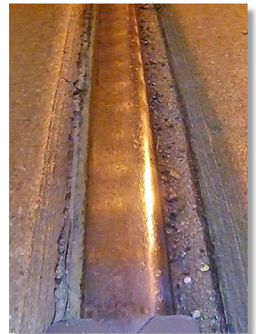
Example of corrugated rail.
