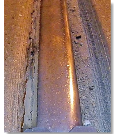
Example of rail surface pitting.
